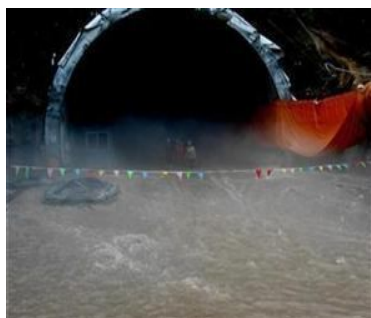
图 6 暴雨后隧道出水情况 Fig.6 Photo of water bursting in the tunnel after a heavy rainstorm
